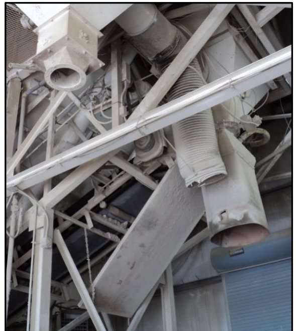
Pictured above are the funnels that dump the required mixture of cement, sand, aggregates, water, and color pigments as needed into the concrete trucks
