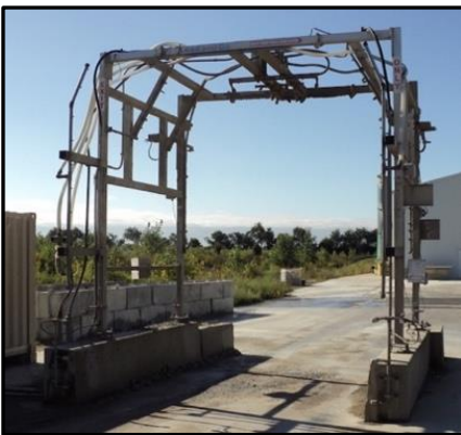
A large truck washing station is located on site
