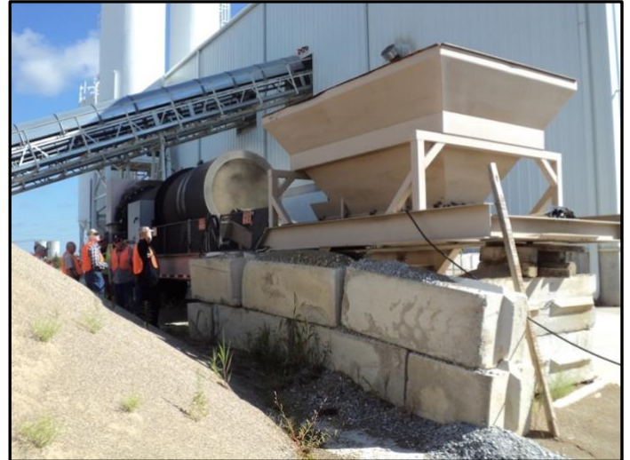
Sand is dumped into a large bin and then runs through a large spinning dryer. Above are the conveyers that delivers the aggregates into the building
